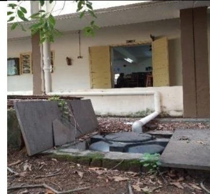
Rain Water Harvesting pipeline – Tank - 3
