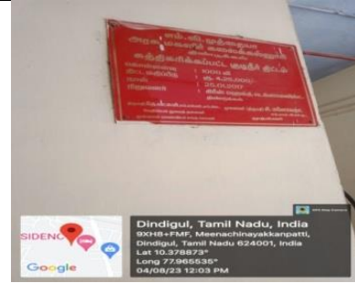
RO - Plant installed by OSA
