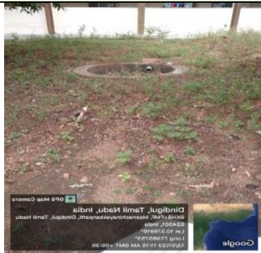
Rain Water Harvesting Pit-5
