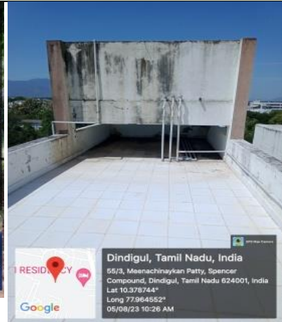
Water Tank in New Building - 5
