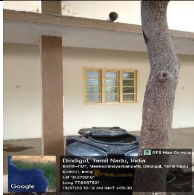
Rain Water Harvesting pipeline – Tank - 2
