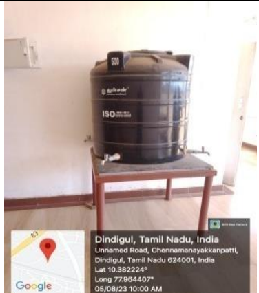
Drinking water Tank - 1
