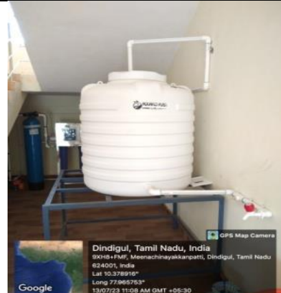
Drinking water Tank - 2
