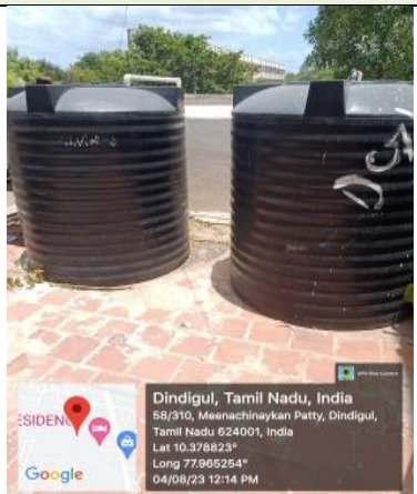
Over head water tank - 7
