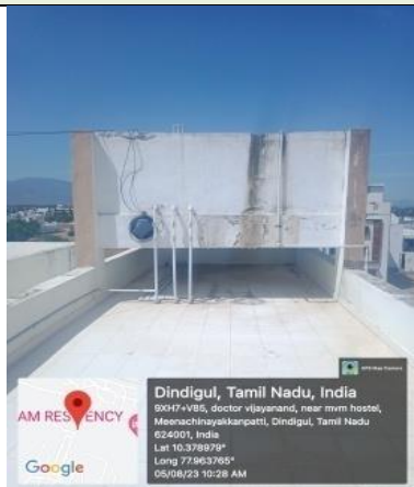
Water Tank in New Building - 6
