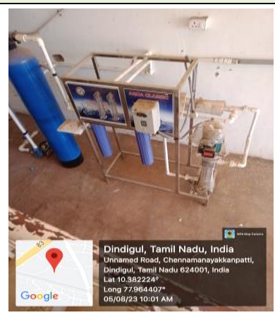
RO - Plant installed by OSA
