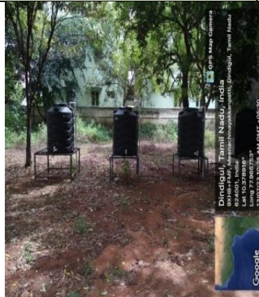
Drinking water Tank - 4
